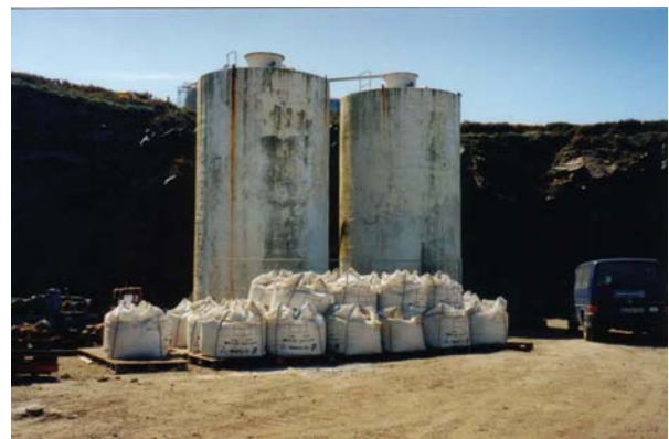
Water Storage Tanks
