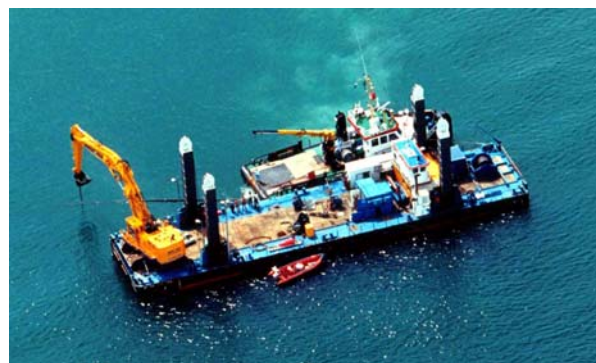
Abeko Server II at Exit Point
