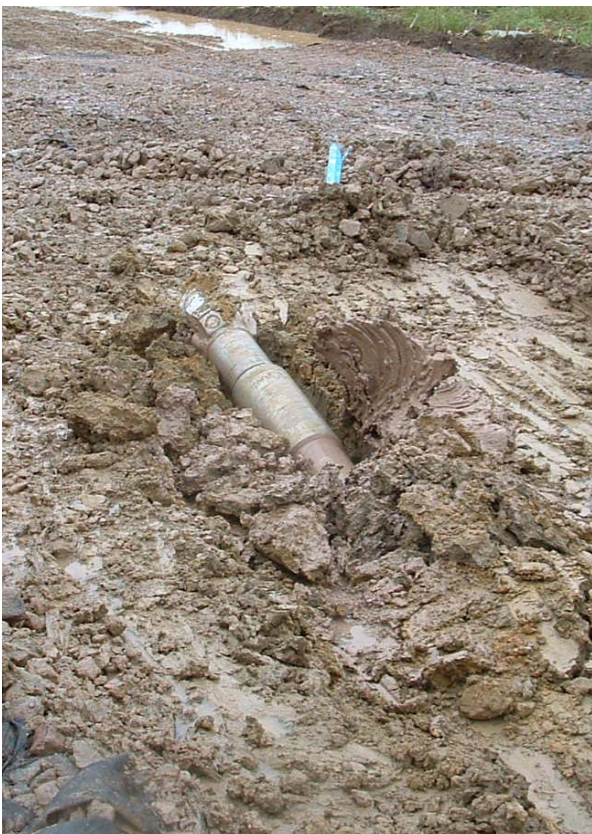
Fig. 2: The 12 ¼" Pilot Bit Breaks the Surface (the blue peg indicates the intended exit point)
